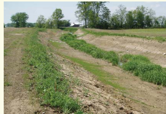
The two-stage ditch immediately following construction. Note the stability of the low flow channel.
